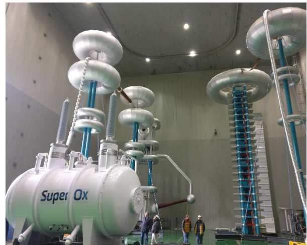
220 kV SFCL at the KERI high voltage test facility
