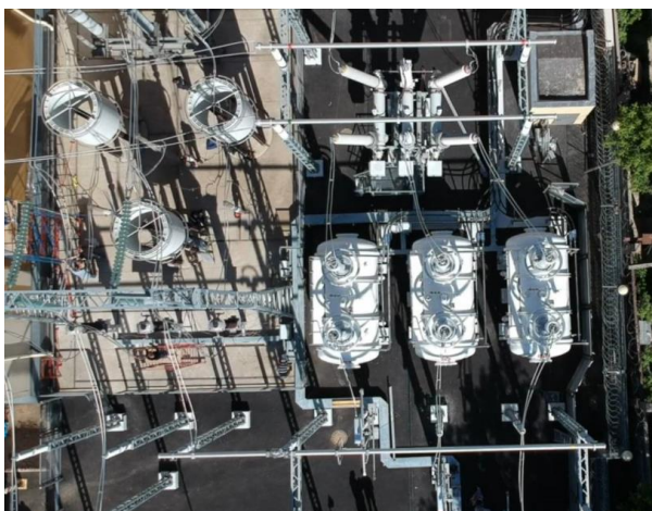
220 kV SFCL at HV substation (ACR and switchgear are visible on the left and top of the picture)
