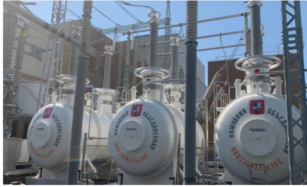
220 kV SFCL at HV substation
